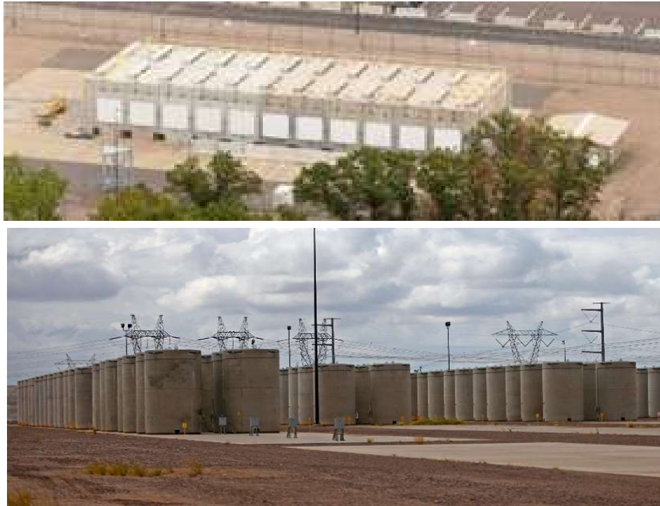
FIG. 6 Examples of storage units comprising horizontal (upper) and vertical dry cask storage systems (lower). (Upper image courtesy of Arizona Public Service/Palo Verde. Lower image courtesy of Xcel Energy).
